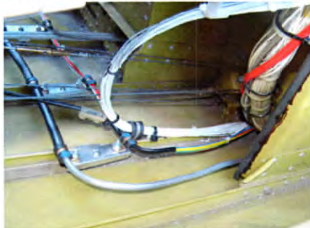
View from tail - right access. Fuel line and electrical secured as described in fig 2. A-A & B-B.
