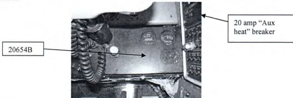
Typical location for 20654B and 20amp breaker.
